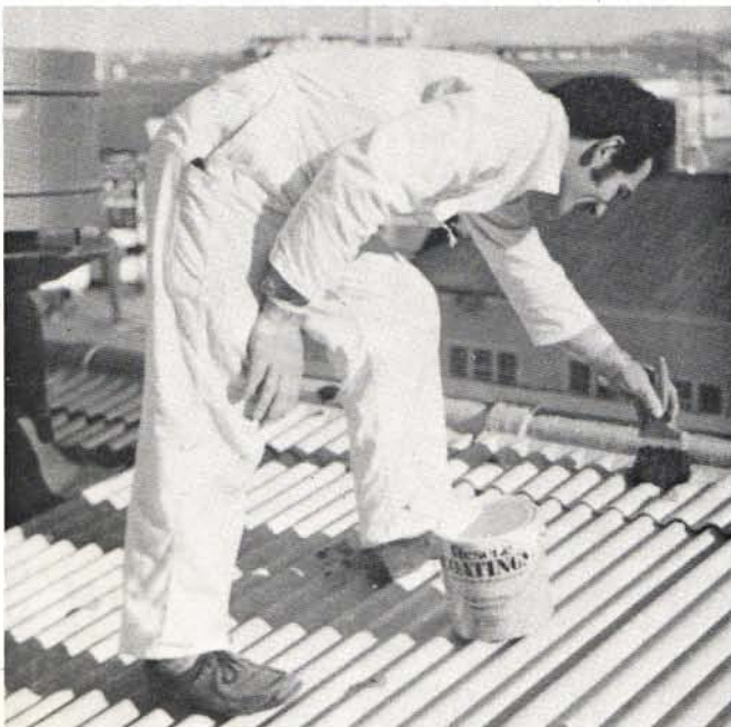
Galvo-One being applied to a roof by Barry Morton of Neville J. Lucas Ltd, Wellington.
