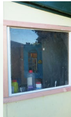
Step four Measure, mark and cut pieces of treated timber to keep window frame in position, as shown. Sand rough edges and fix with galvanised nails.
