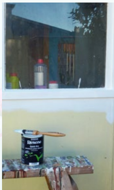
Step six Wash any existing painted areas and, once dry, prime the window frame and bare wood with one coat of Resene Quick Dry. Allow two hours to dry.
