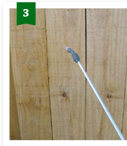
Apply a generous amount of the diluted solution across the fence, working it into the wood using a stiff-bristled brush. Leave for 48 hours. Wash off.
