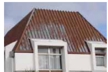
Almost certainly a primer was not used on this roof or the garage door on the next page.
