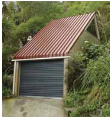
An example of longrun (or tray section) roofing.
